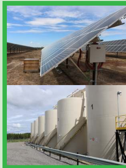
Fort Chipewyan Power Generation Diesel + Solar
