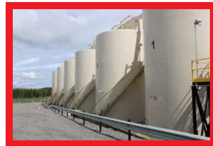
Fort Chipewyan Power Generation Diesel Only
