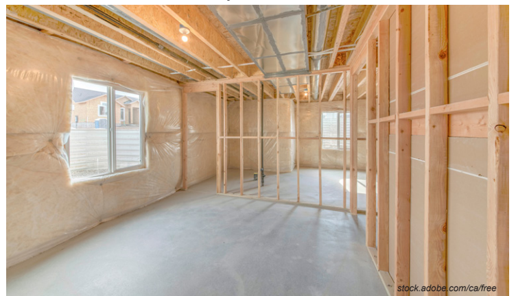
The outside wall has a thick layer of insulation with vapour barrier
