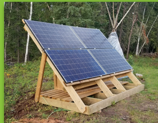
Solar Array Unit from the front
